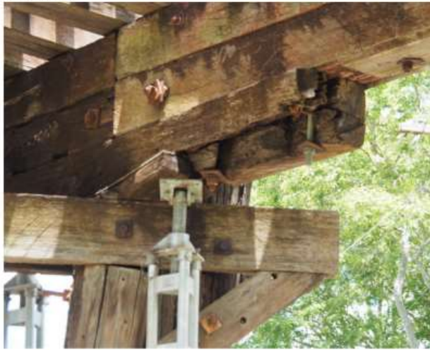
Figure B-14 Terania Street – Rotten and damaged east corbel at Pier 6 (Source: FBE)
