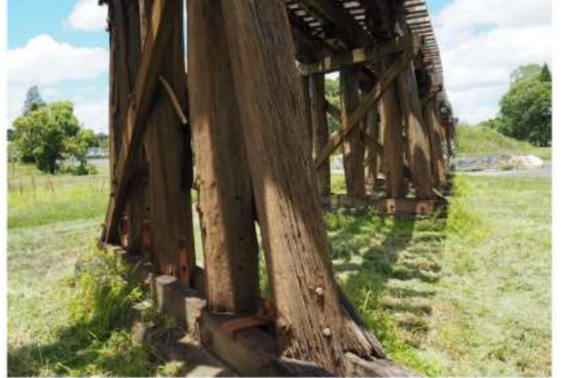
Figure B-15 Terania Street – Splitting & weathering of piles at Pier 11 (Source: FBE)
