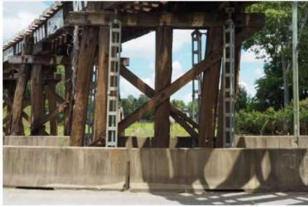
Figure B-13 Terania Street – Evidence of global rotation of Pier 6 together with failed pile (Source: FBE)
