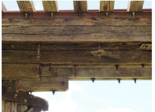
Figure B-16 Terania Street – Loose connections & weathered beams (Source: FBE)
