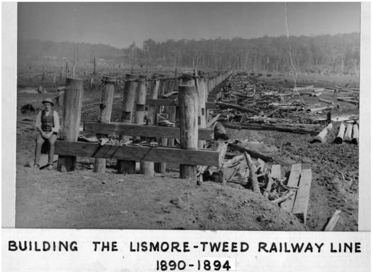
Figure 1.7 1890s image showing clear felling of local timbers at Lismore, in the immediate vicinity of timber bridge construction that was underway. Source: Construction of the Lismore – Tweed Railway Line, c1890s sourced from the Richmond Rivers Historical Society, Folder Transport – Railways, image 52 as cited in Extent Heritage, 2017, Lismore Underbridges (UBN62837A & UBN62837C) Interim Statement of Heritage Impact FINAL , prepared for John Holland Rail Pty Ltd, p26
