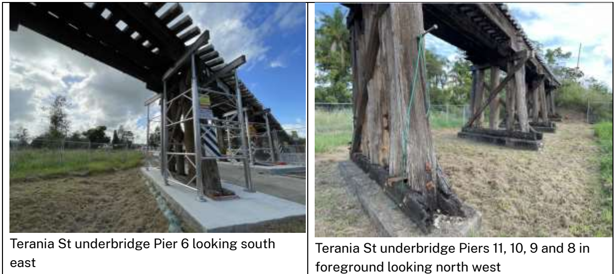
Figure 1.10 Terania Street underbridge showing condition. Source Bridgedoctors September 2023
